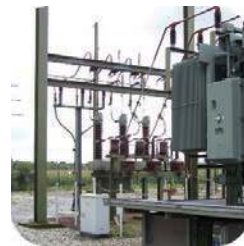
Power Transmission and Distribution
